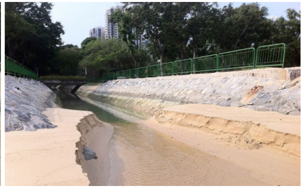
Fig. 255. Location 4: In March 2017, the blockage was cleared by a mechanical digger. (Photograph by: G. J. H. Oliver).
